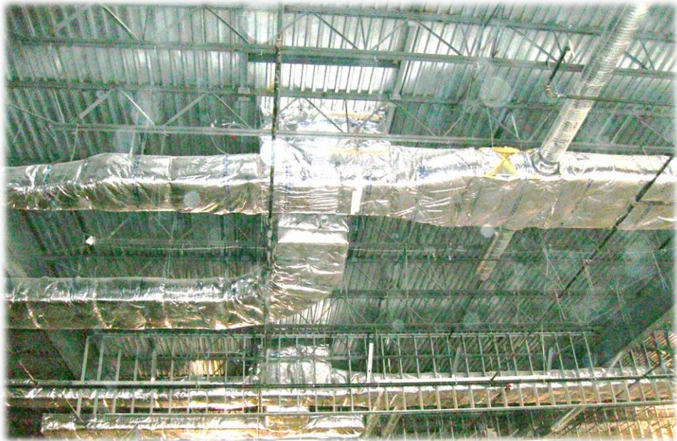
(above picture: commercial heating/duct work)
