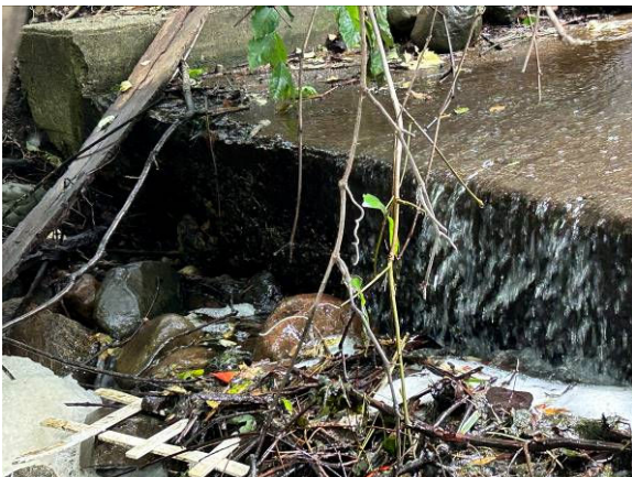
Photo 24: Right side of apron showing sparse rip rap, voids with seepage, and woody debris.
